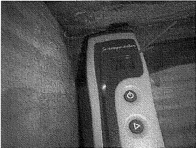
Item 10. Moisture staining on band joist under den/office window. 18.4%
