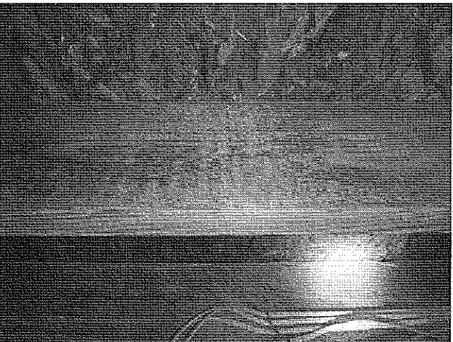
Item 7. Areas of mold on floor joist in basemetn area.
