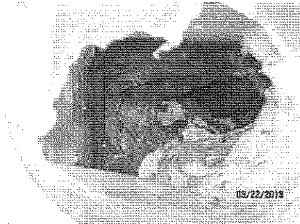
Exposed Wall Cavity Wood Rot and Mold Like Growth
