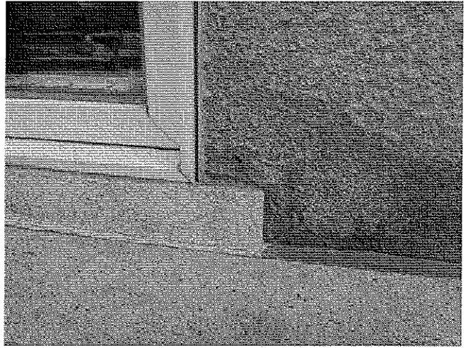
Item 1. Moisture staining around windows.
