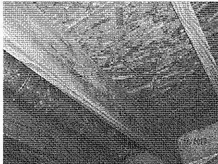
Mold Like Growth on Joist. No Water Source Detected in the Area, Possible Pre-Construction Growth.
