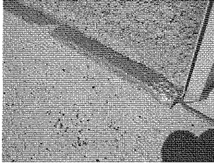
Exposed Opening in Stucco
