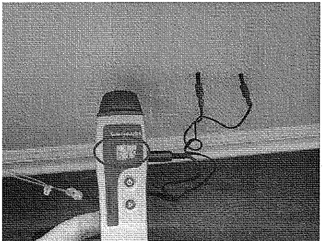
Item 11. Moisture test under master bedroom window. Middle of window.
