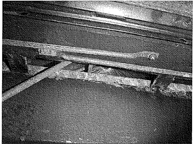
Item 6. Basement fire place firebox showing signs of issues with moisture.
