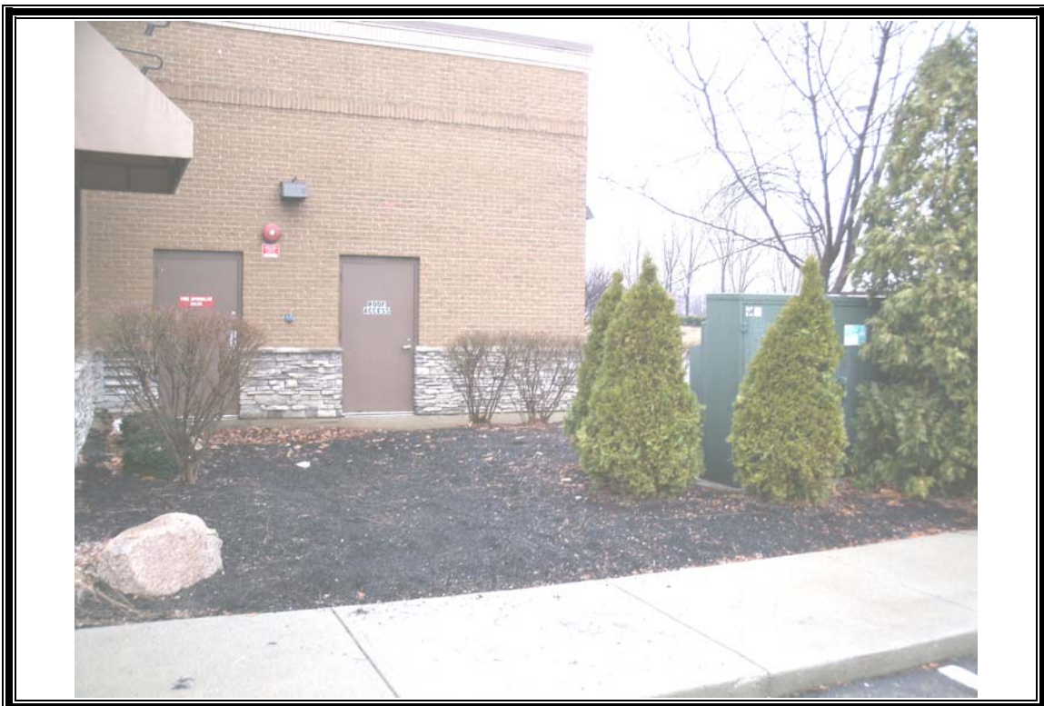
Photo 4: March 10, 2010 Mulch area containing the apparent grease trap cover. A pad-mounted electrical transformer is shown to the right.
