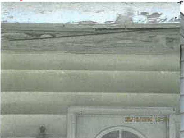
Rotting wood on porch roof.
