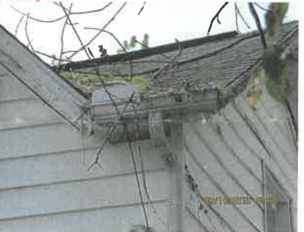
Gutters full of debris.
