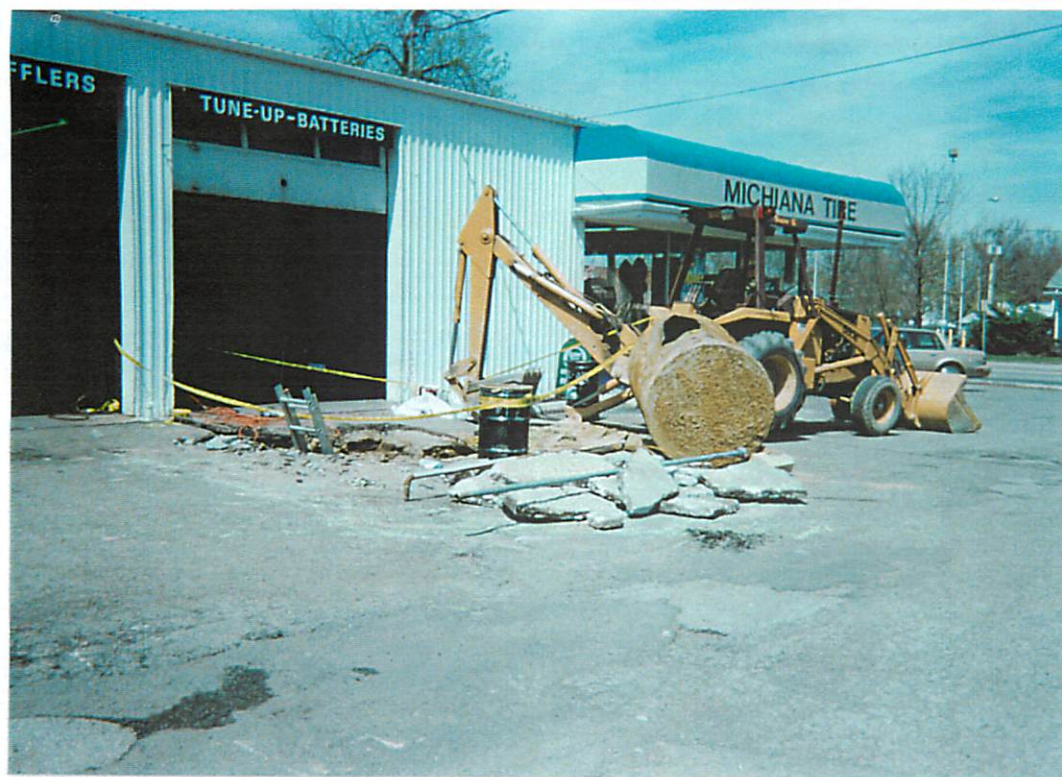
View of tank pit after removal of the used oil UST. Note: deformation caused by UST removal operations. (view to Northwest)
