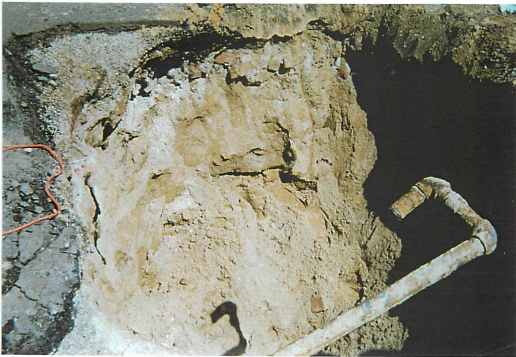
View of north wall of UST excavation. Note fill pipe from west, and brick/concrete foundation.
