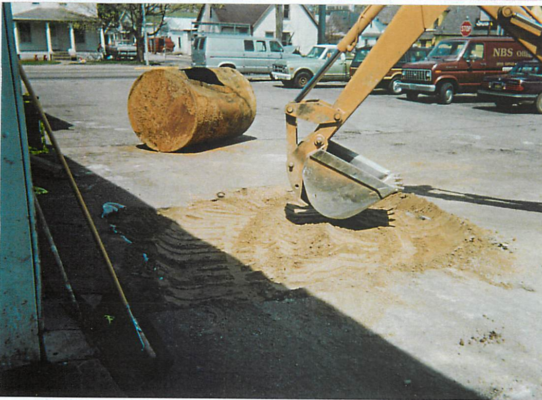
Excavation backfilled to approximately 6" below grade. Excavation was finished to grade with #304 stone (view to Northeast).
