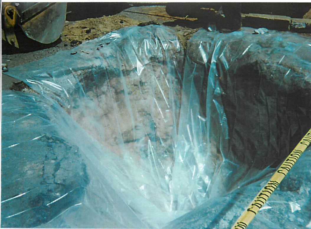
Former used oil UST tank pit lined with 6-mil poly ethylene sheet prior to backfilling (view to Northeast).
