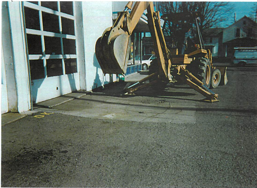
Site conditions prior to excavation activities. Used oil UST is located beneath the concrete pad. (view to North)
