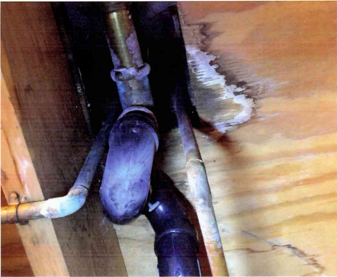
Moisture staining below master bathtub.
