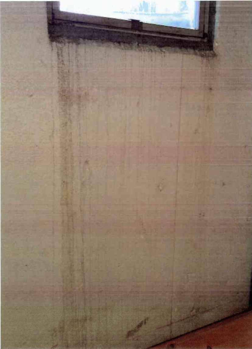
Moisture staining at E basement window.
