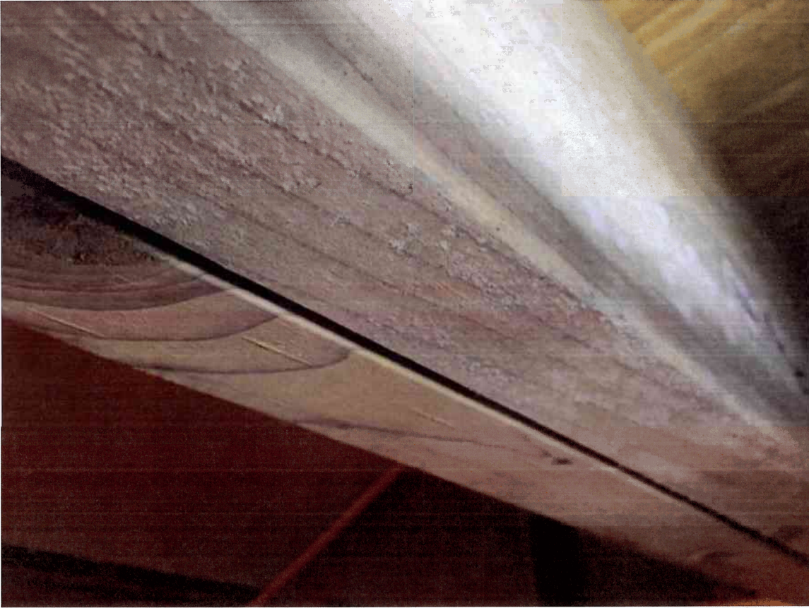
Fungal growth in basement.
