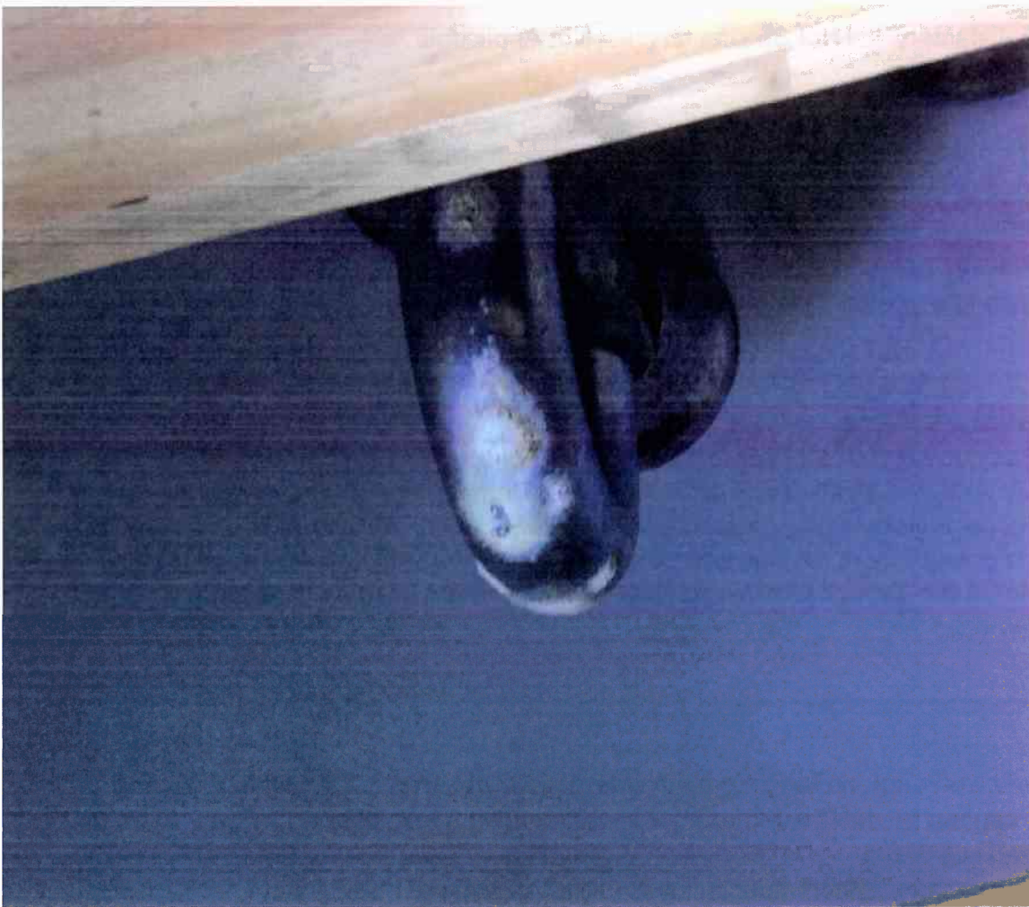
Hall bath sink drain deterioration.
